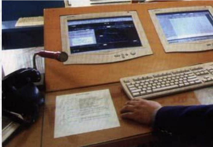
Wireless dispatching telephone in a station
